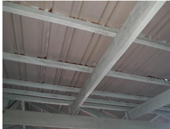
Nikao Panama Recreation Centre – Rust spots and holes in the roof.
